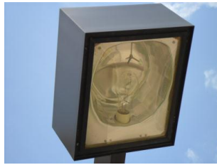
Before 400w Metal Halide
