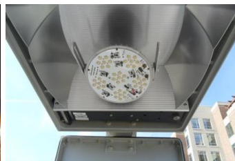
400 Watt Retrofit Parking Lot Hospital
