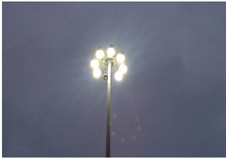
Hi Mast Triple 93 Watts 1000W To 279W Train Switching Yard
