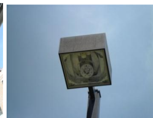
400 Watt Retrofit 93 Watt University
