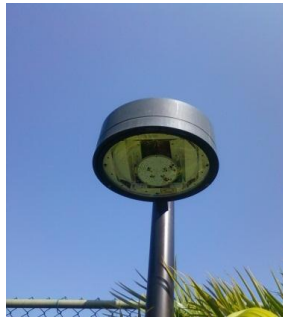
400 Watt Retrofit 93 Watt Shopping Center Hawaii
